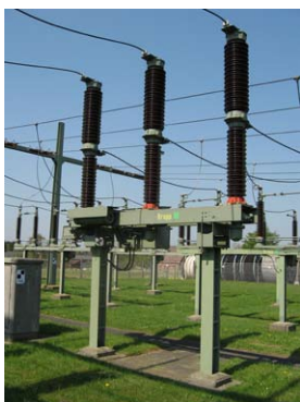
Foto of the power switch
